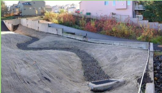
Two bioswales for a housing development. Foreground - under construction; background - established (Source: Wiki Commons)
